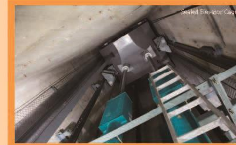
Sealed Elevator Cage
